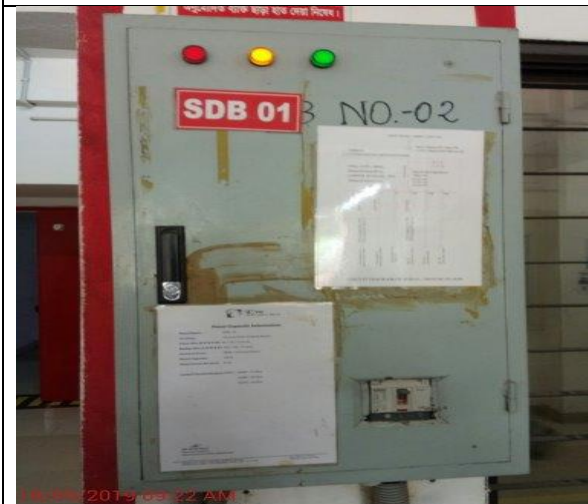
Electrical switch/box with cover & warning signs
