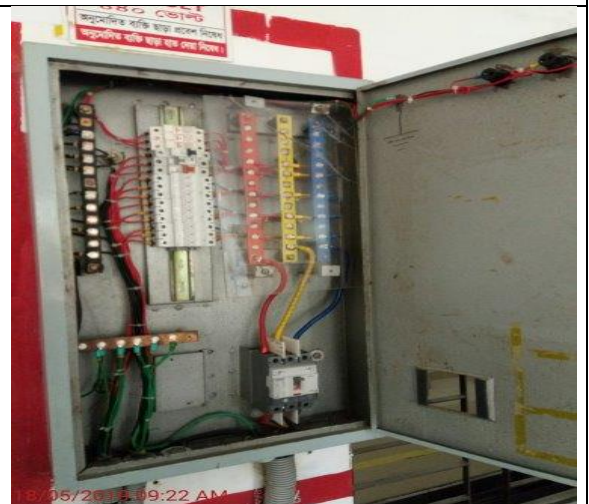
Electrical box cabinet with wiring
