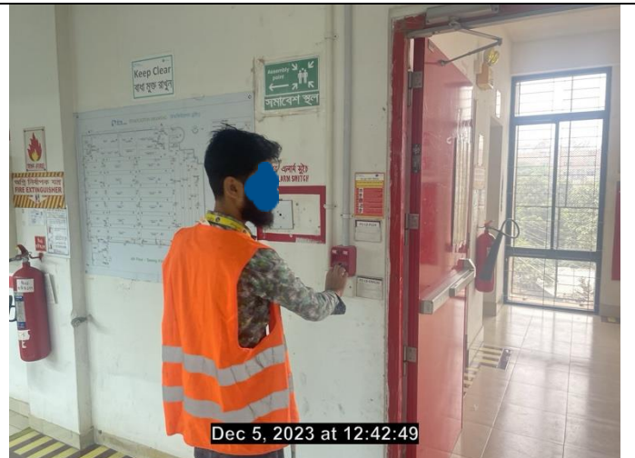
Fire alarm call point live testing
