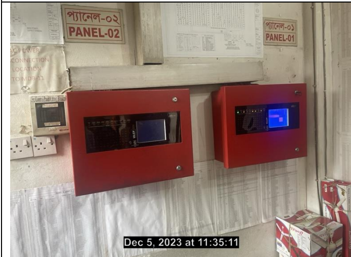
Fire control panel
