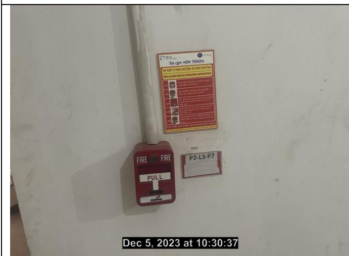
Fire alarm call point
