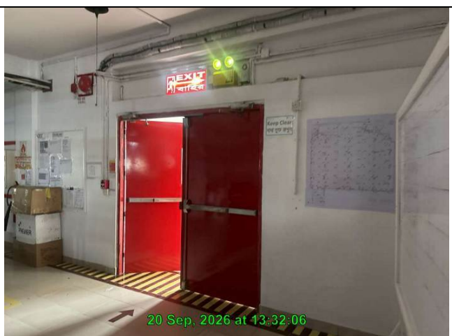
Fog light Checking with IPS back up
