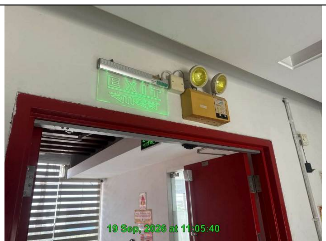
Illuminated exit sign
