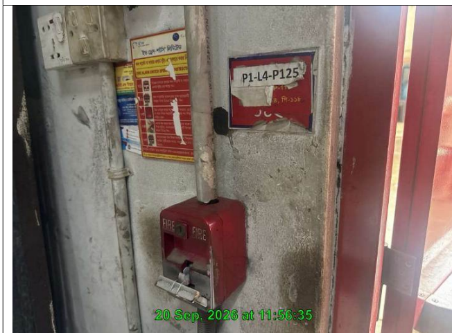
Fire alarm switch
