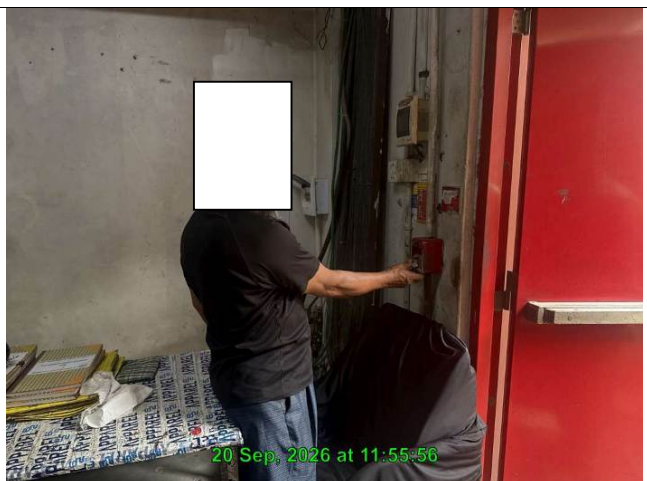
Fire alarm call point live testing
