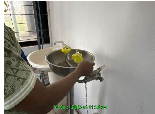
NC_3.4.5 (e): Eye wash station was not properly working.
